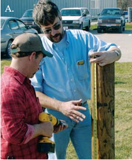
Constructing a permanent fence that may last over 40 years is a job best done once and done right. Be sure that enough time and thought is given to the planning stages.
