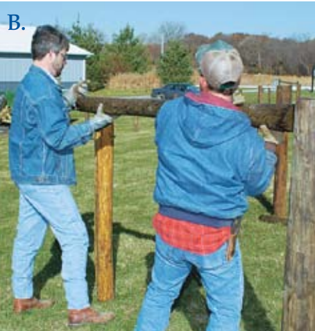
Installing Brace Post, 8 ft. (inside to inside) down fence line from end post.
